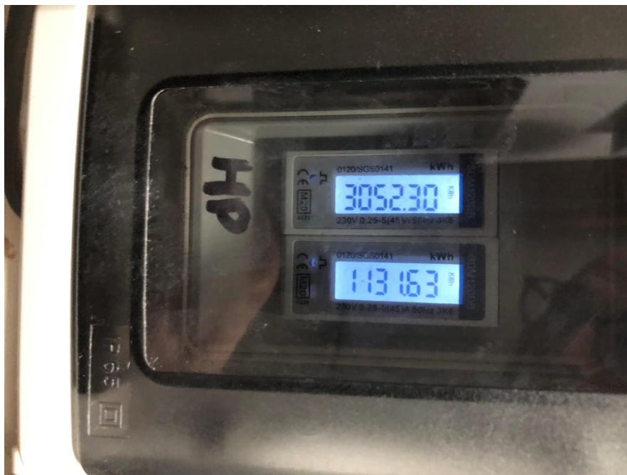
Figure 10: Electricity meter, showing ASHP consumption at the top
