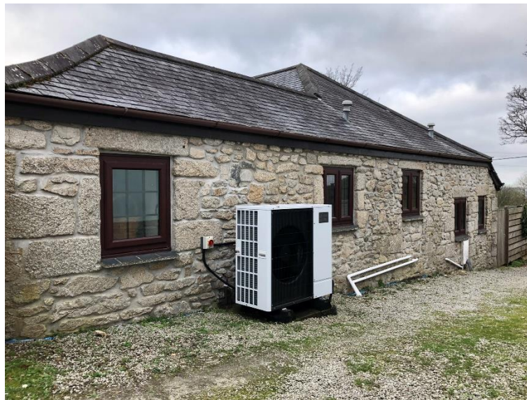
Figure 33 - Plough Court, monobloc AHSP located on old oil tank plinth
