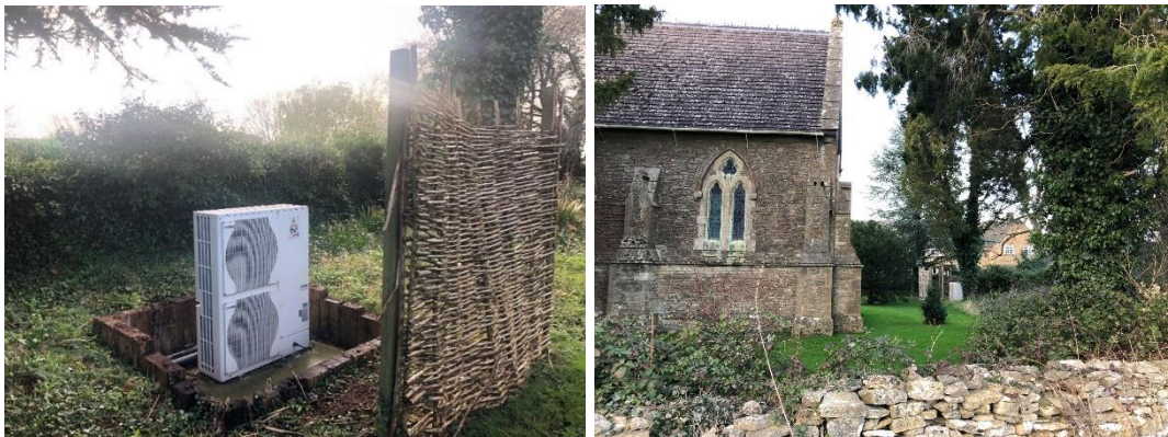
Figure 29 - ASHP external unit location, Left: close-up, Right: View from rear of grounds
