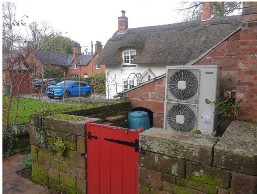
Figure 12: ASHP at rear of property
