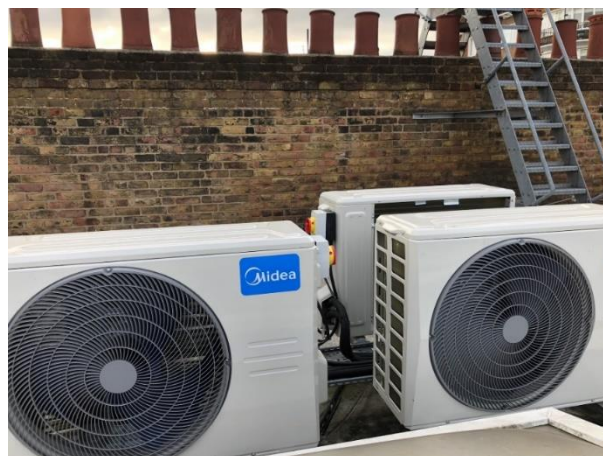
Figure 22 - ASHP units installed on the roof
