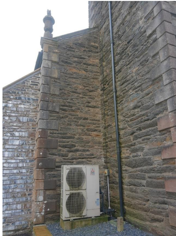
Figure 17: Mitsubishi Zubadan ASHP Unit at St Anne's
