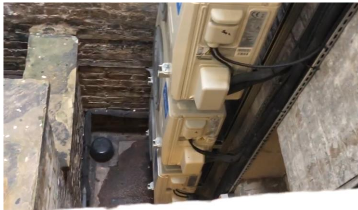
Figure 23 - Wall mounted external units, with poor access and close proximity to neighboring windows
