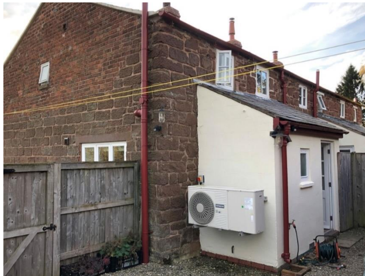
Figure 7: ASHP installation at rear of property
