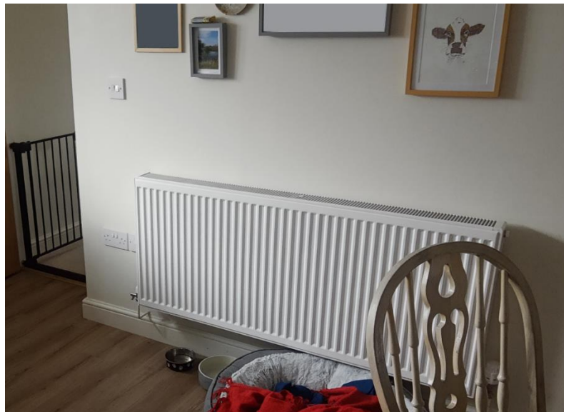
Figure 8: Kitchen radiator with 10mm connecting pipework
