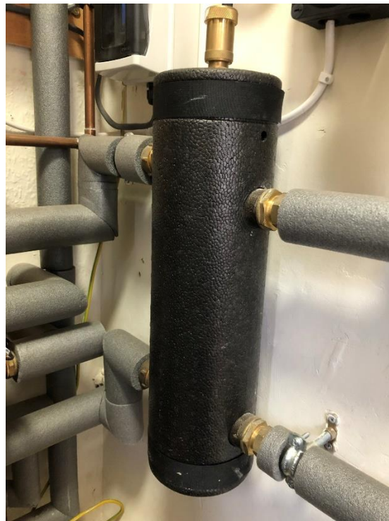
Figure 9: Low Loss Header in the plant room
