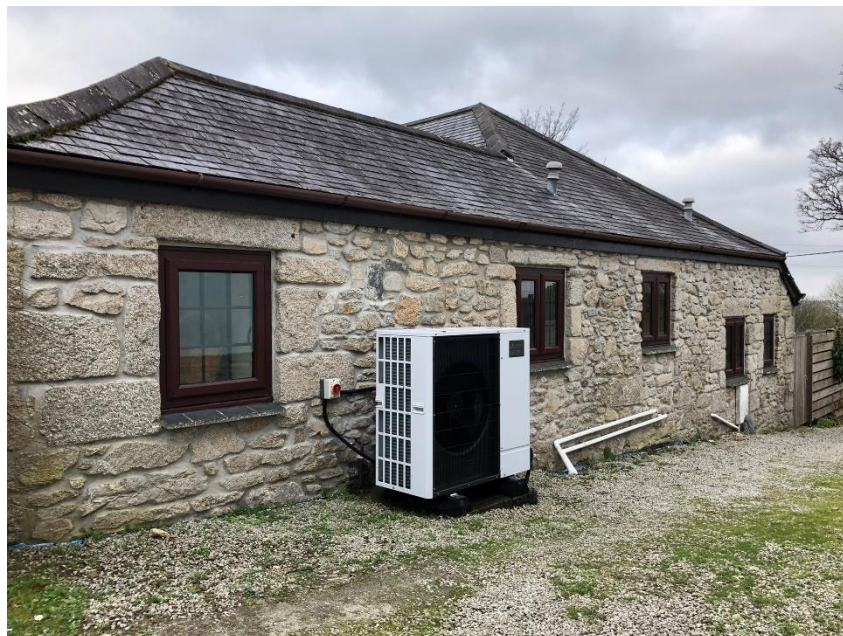
Figure 34 - ASHP installed on the side of the property
