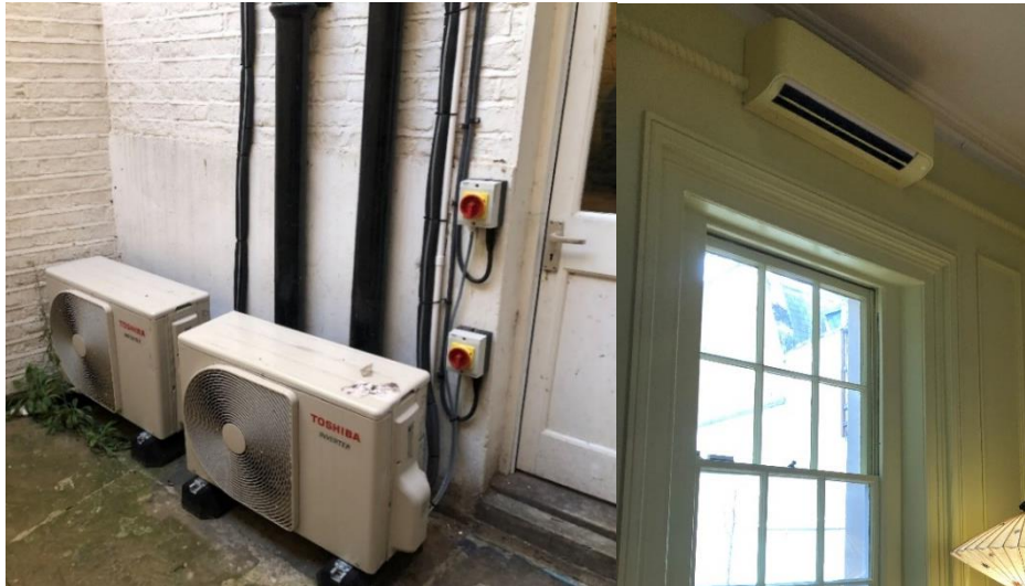
Figure 20 - ASHP installation at Elizabeth street. Left- External Units. Right- Internal unit, painted to match the internal décor.
