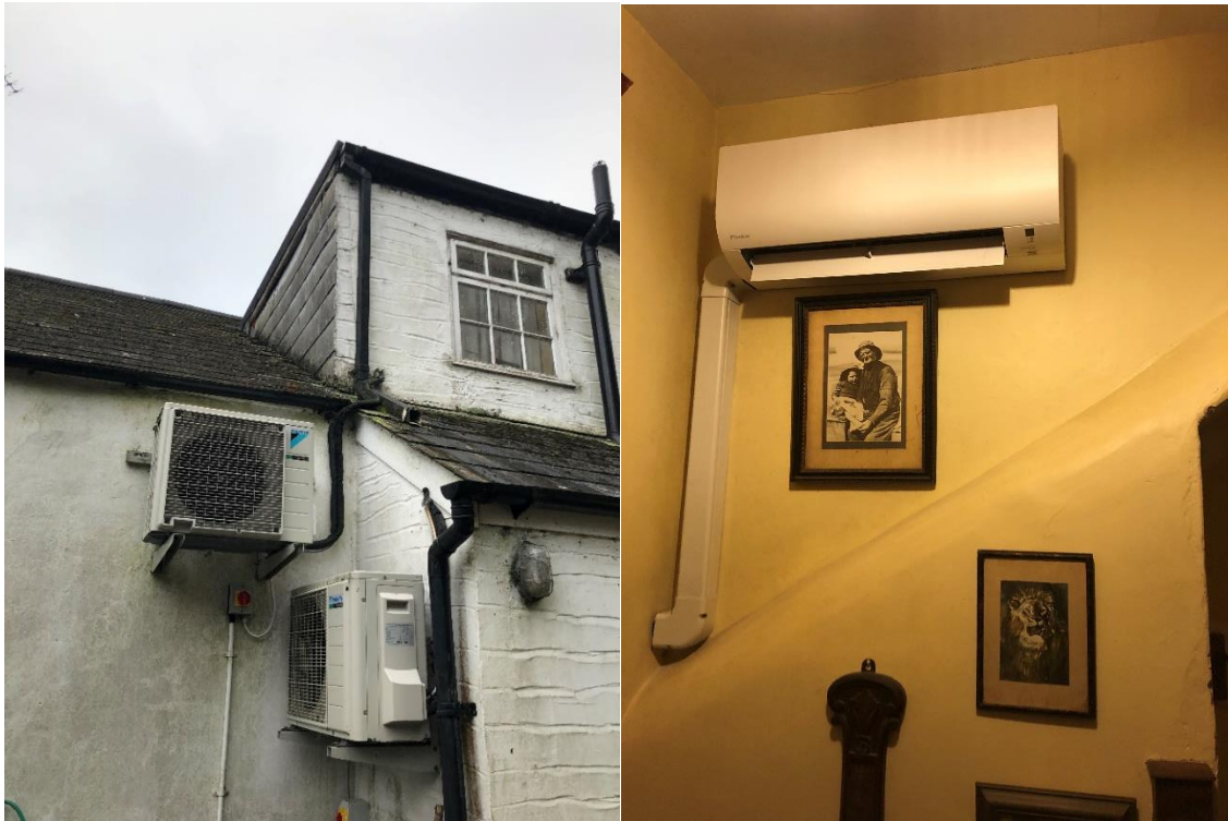
Figure 32 – Left: ASHP units installed on the side wall of the property. Right: hallway condenser unit
